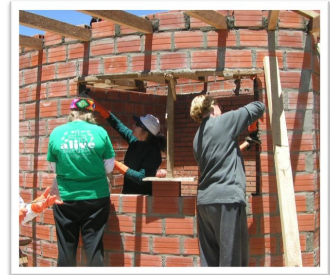
Volunteers work to build an addition to a clinic in Bolivia. Volunteers help support our programs abroad and our headquarters in Raleigh, NC.
